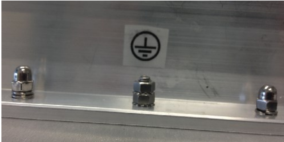
Figure 44: 9502 Protective earth grounding
